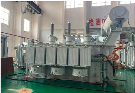
Transformer type: SFZ-30000/66Client: COBRA ChileFactory Acceptance Test
