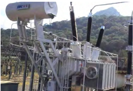
Aibania Capacity 60MVA voltage ratio 242KV/10.5 KV
