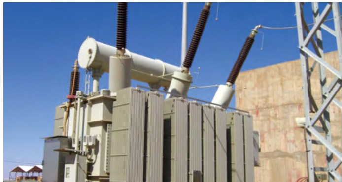
China National Gold Group OSFZ-125000-220 transformer
