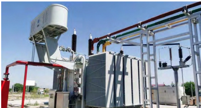
Main transformer SFZ11-63000-110, Samarkand Steel Works, Uzbekistan
