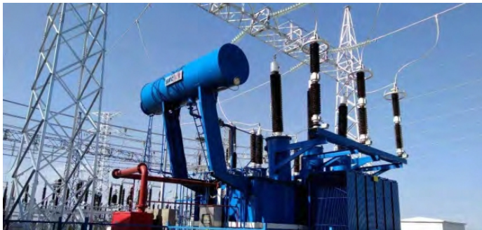
OSSFZ-125000/230 transformer from Kyrgyzstan
