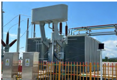
SFZ11-100000/110 Power Transformer
