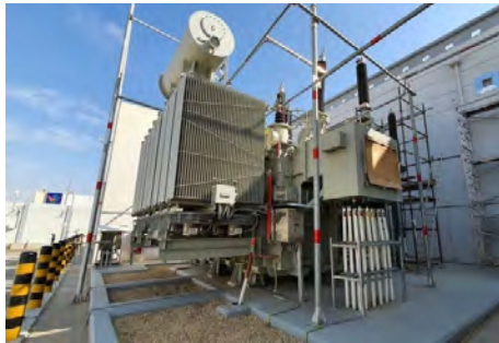
Australian VISE paper SFZ1-31500-132 transformer
