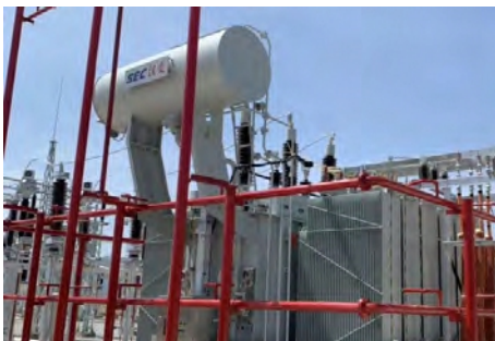
SFZ11-63000-115 transformer for TASC049MW photovoltaic power station in Vietnam
