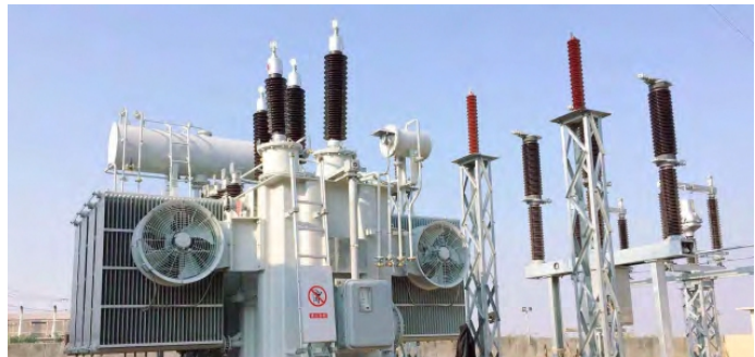
Pakistan SFZ11-26000/132KV transformer
