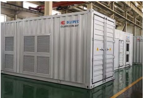
Photovoltaic Box Type Booster Station
